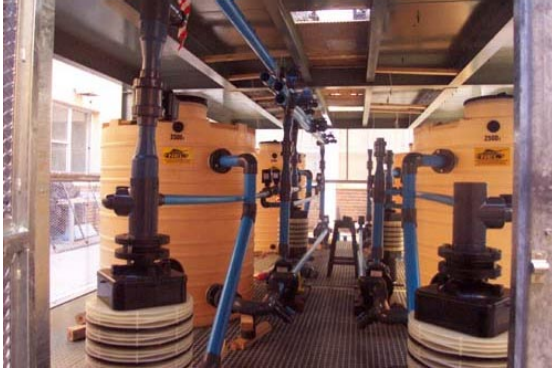
Fig 5. Lower level of VRB installation
